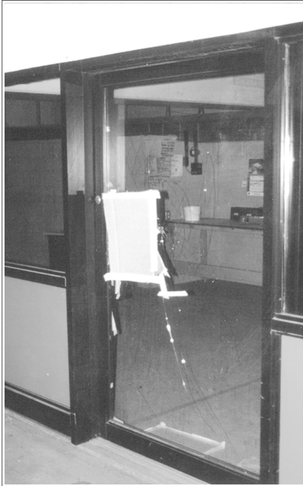
If prompt attention is not given to maintaining a property, it can contribute to a sense of fear.
