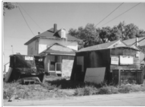
Poor maintenance and neglect of a property provides a feeling of an unsafe place.
